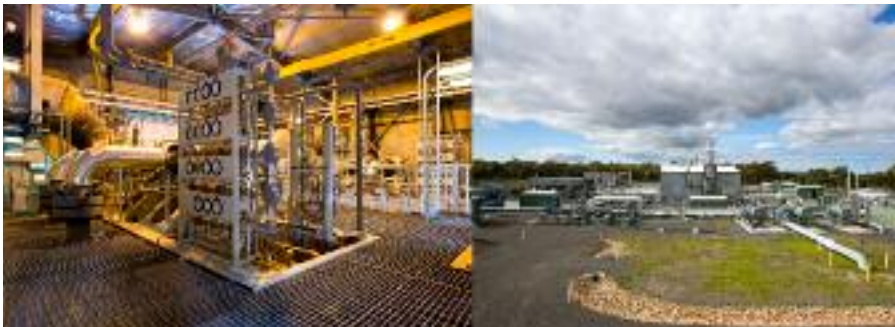
FIGURE 1.2. An Australian high-pressure pipeline compressor station control room (left) and view of the overall installation (right).
