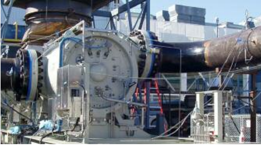
FIGURE 2.2. Typical gas turbine driven compressor during a field performance test.
