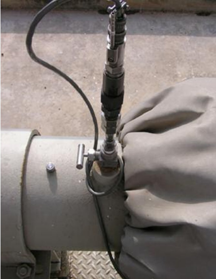
FIGURE 4.5. High-frequency pressure transducer in discharge pipe.
