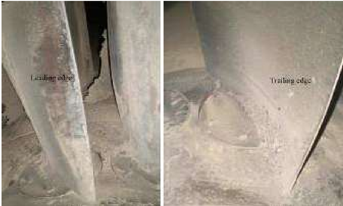
FIGURE 9.2. The authors assessed the impact of erosive particles on the studied fan after 9,000 hours' in-service operation. The blade leading edge profile was compromised and outlet guide vanes had lost almost half their chord, left. There is also evidence of erosion on the blade pressure surface in the hub region, right.
